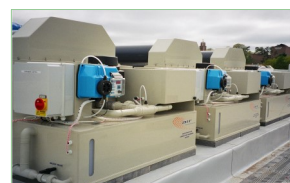
REMOTE ROOF MOUNTED SCRUBBERS
